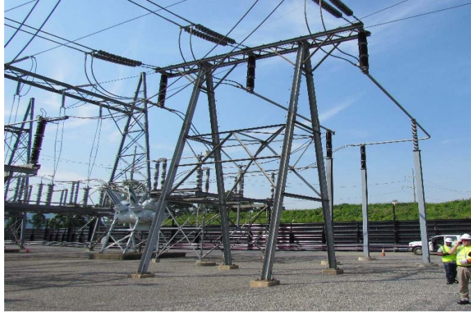
Image 6: Typical A-Frame Deadend Structures
